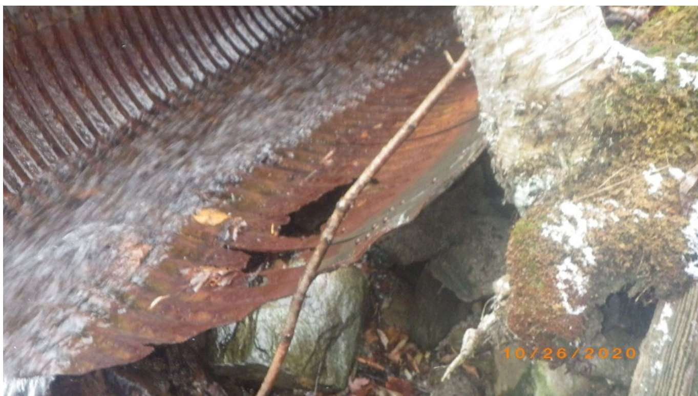
Picture 4: Deteriorated Invert
