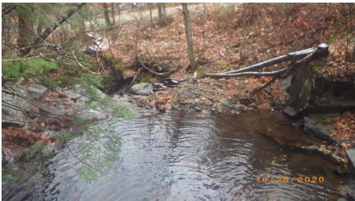
Picture 6: Scour pool downstream of Bridge 29
