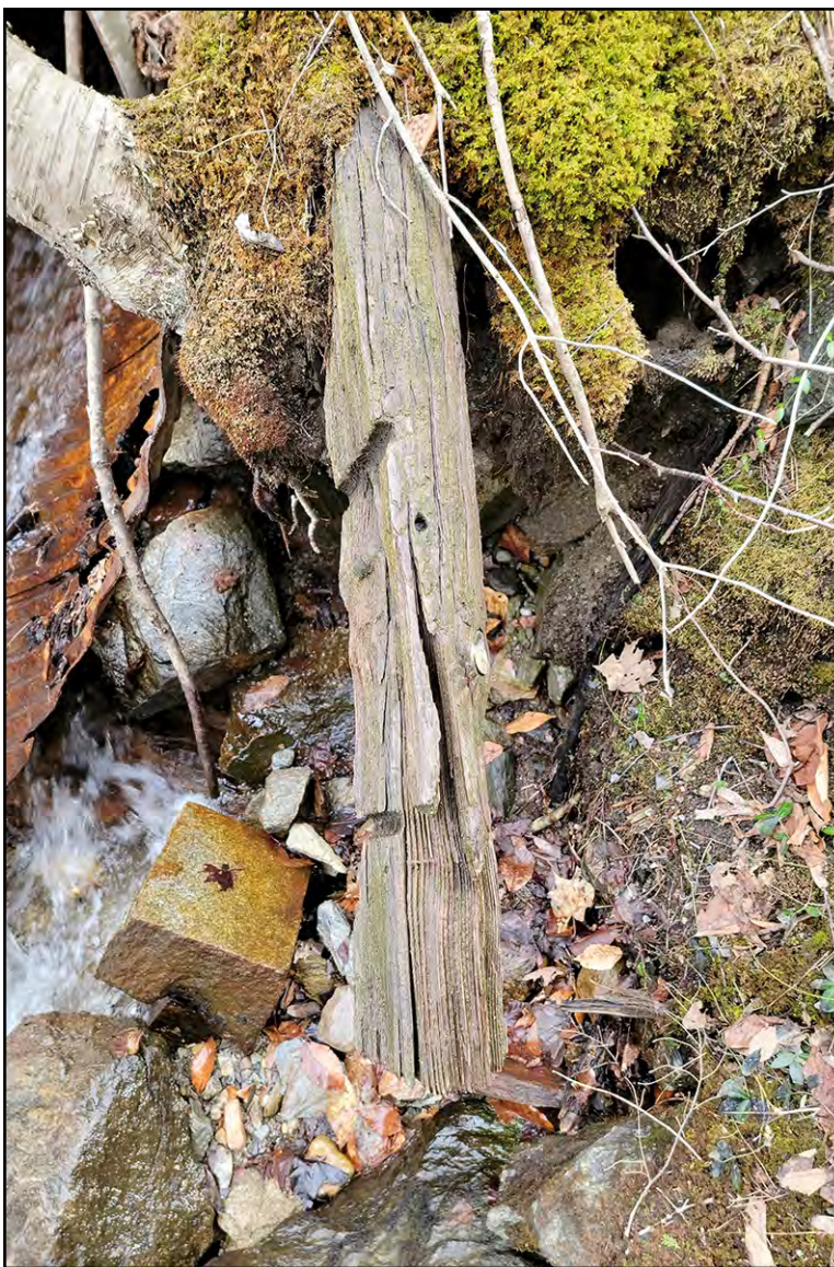
PLATE 3: Closeup of Beam Protruding from West Side of West Culvert Exit, View East
